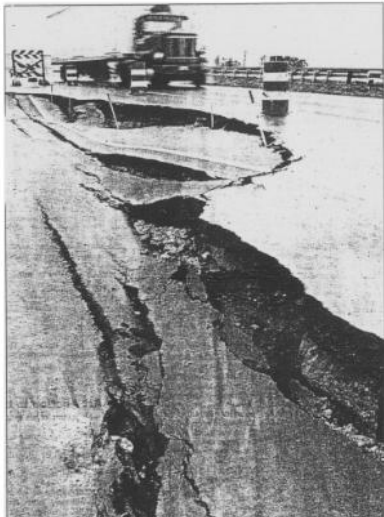
DAMAGED FREEWAY: A truck passes the damaged section of the Durham Freeway near Hillandale Road. A section of Durham's newest
